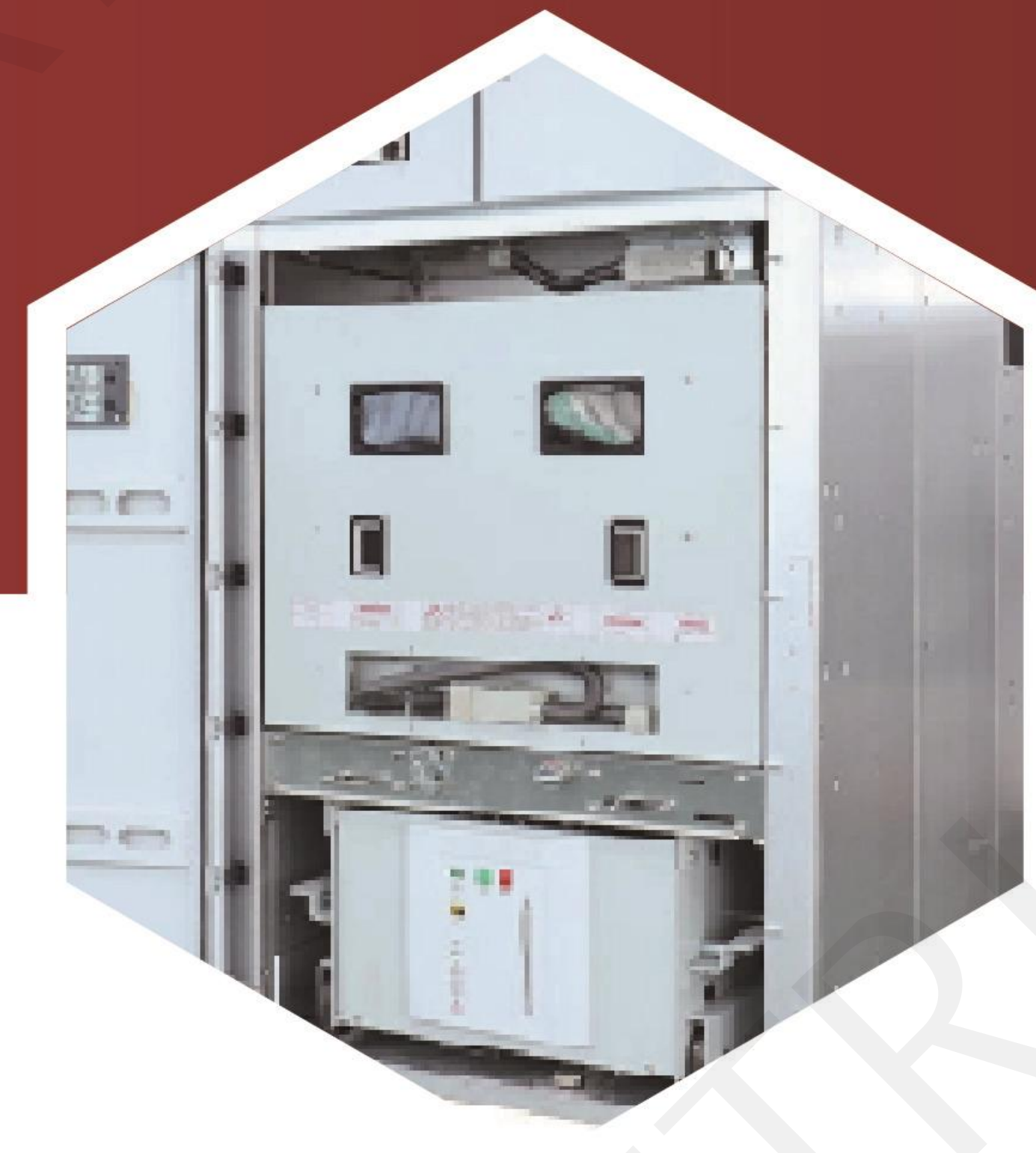
Withdrawable Circuit Breaker Compartment
